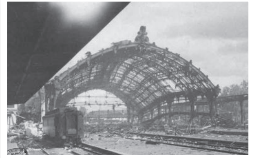
Dijon train station glass roof after the sabotage by the German army
